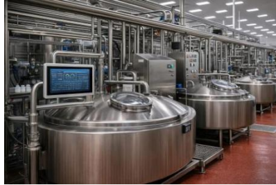
Dairy & Beverage Production Line
